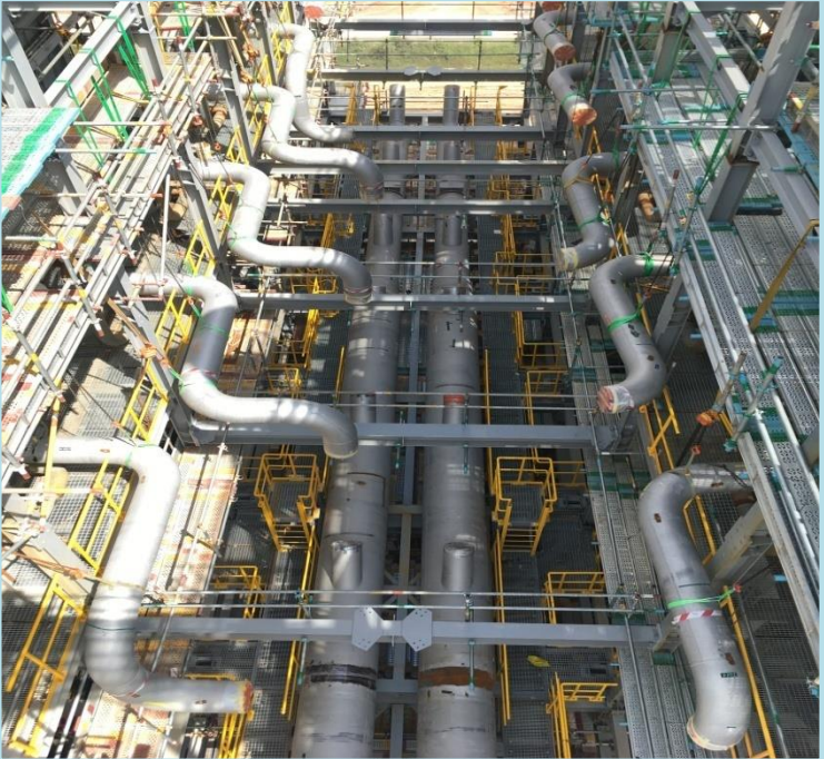
➤ Furnace Pipe Spool welding daily progress average 300 dB by our Welding Team
