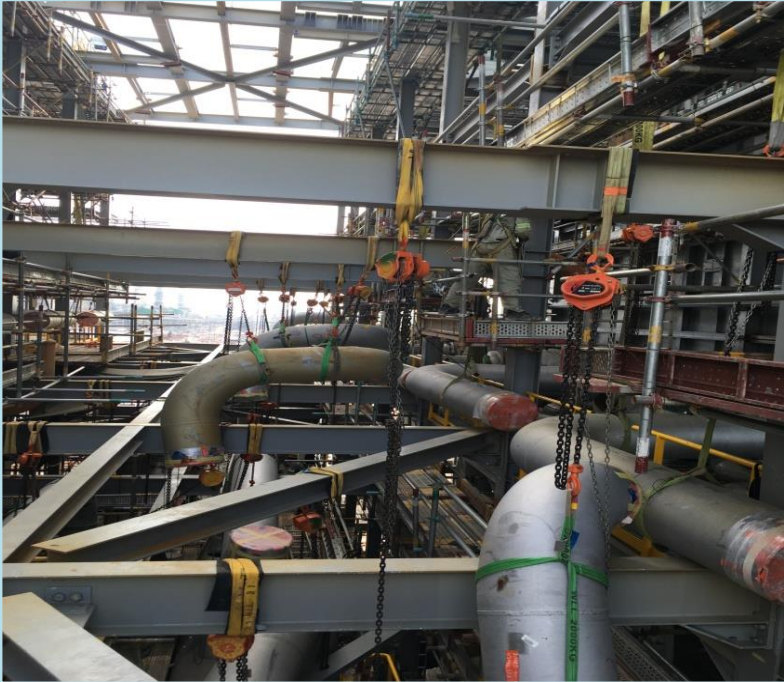
➤ Pipe Spool launch by Lifting Team of more than 100 spools per day
